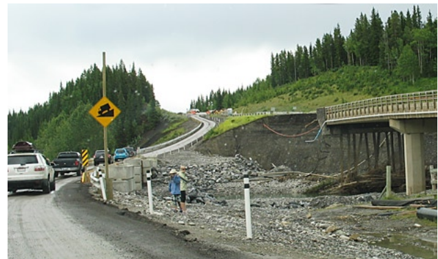
Temporary bypass around the washed out Highway 66 Bridge over the Elbow River east of Allen Bill Pond.
