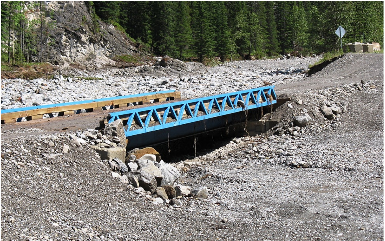
Flood deposits filling Canyon Creek channel at the bridge on Canyon Creek Road. Upper photo taken August 2009. Lower photo taken August 2013. Note tree roots dangling from bridge and gravel packed into triangles: evidence that the bridge had been inundated during the flood, and cleared by road crew prior to this photo being taken.
